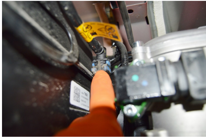
(Fig. 6) This is another view of the return line showing the quick connect coupling.
