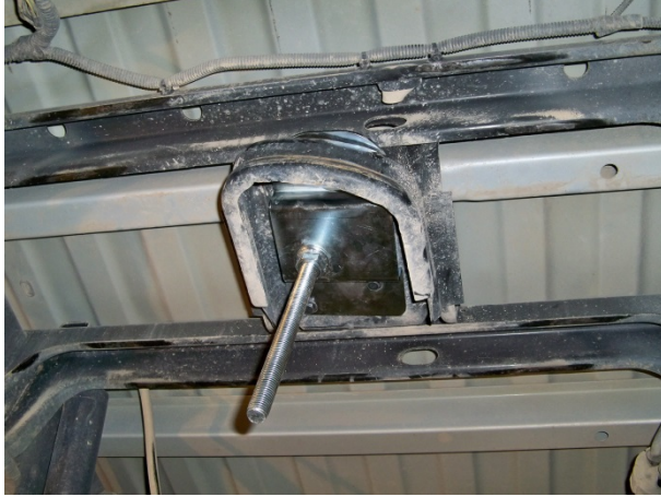
(Fig. 2) Cross member in 03-12 RAM vehicles showing STAFS top Truck Mounting Plate and Threaded Rod installed.
