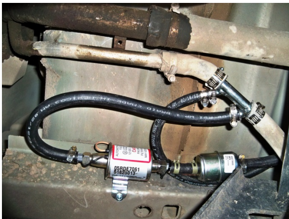
(Fig. 15) Vent Fill Neck Adapter installed.
