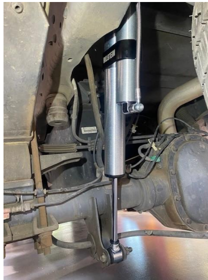
Figure 2. Rear Driver Side without wiring harness (View from rear)
