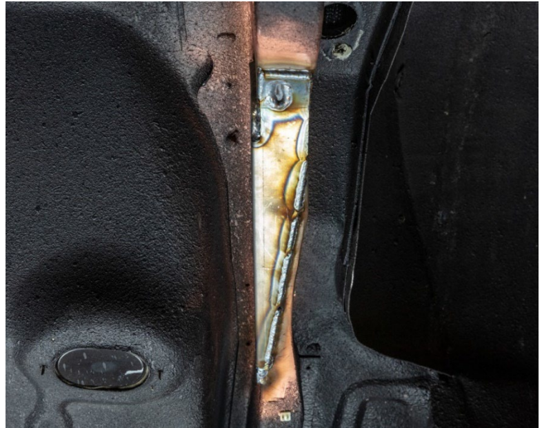
Figure 3: Two images of the raw metal on the frame rail
