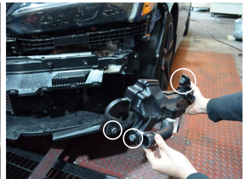
9. Remove the three bolts securing the intercooler pipe resonator, then remove the resonator.
