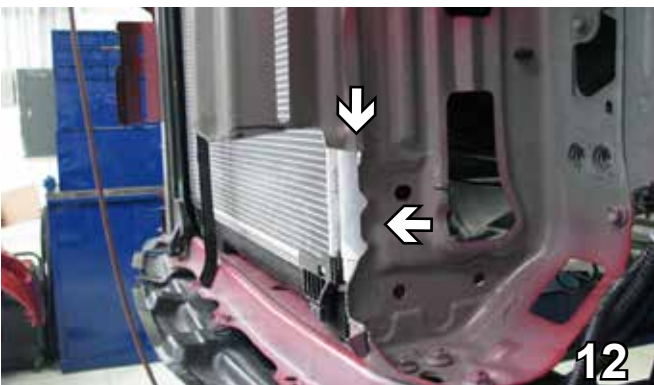
12. Showing the lower frame support webbing after the trimming has been completed.
