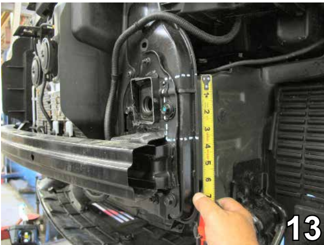
13. On the driver's side radiator support, mark and trim a section 3 1/2" high and flush with the frame rail to open the area for baseplate installation.
