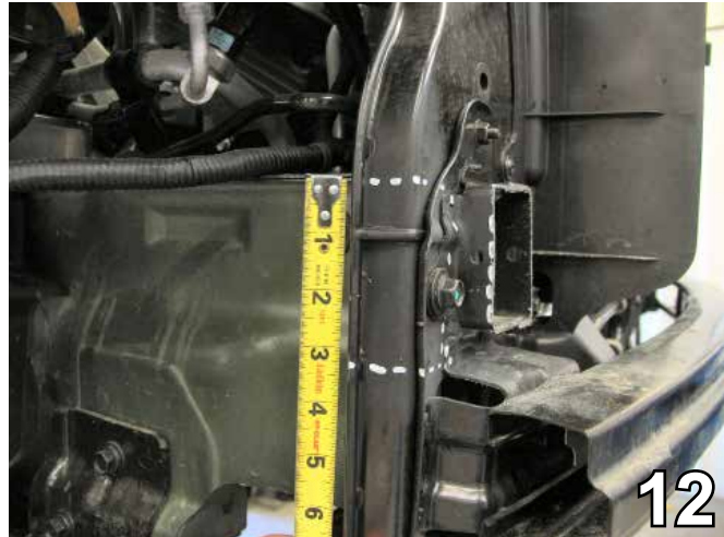
12. On the passenger's side radiator support, mark and trim a section 3 1/4" high and flush with the frame rail to open the area for baseplate installation.
