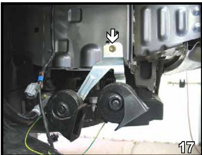
17. Disconnect the horn wiring and, using the 12mm socket, remove one metric bolt from the horn bracket. Set horn bracket and bolt aside to be reinstalled later.
