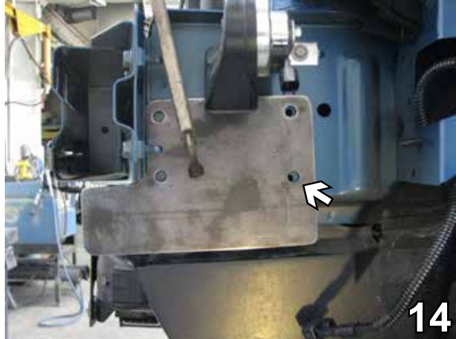
14. Align the baseplate with the existing hole. Clamp across the top of the frame with the large vise grip. This is done on both sides of the vehicle.
