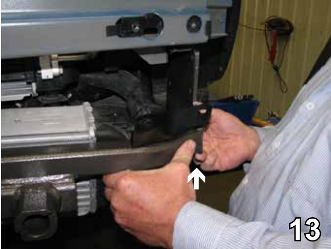
13. Continue to move the baseplate and the turbo on up into position. This is done on both sides of the vehicle.
