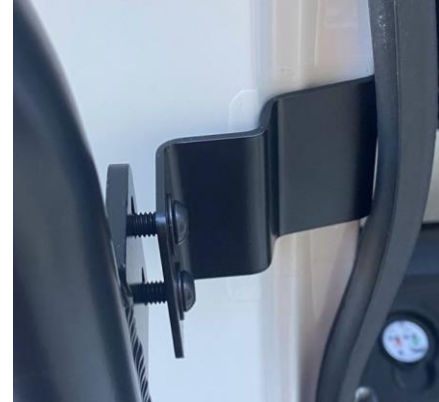
Figure 16: Example of gap between bracket and rack
